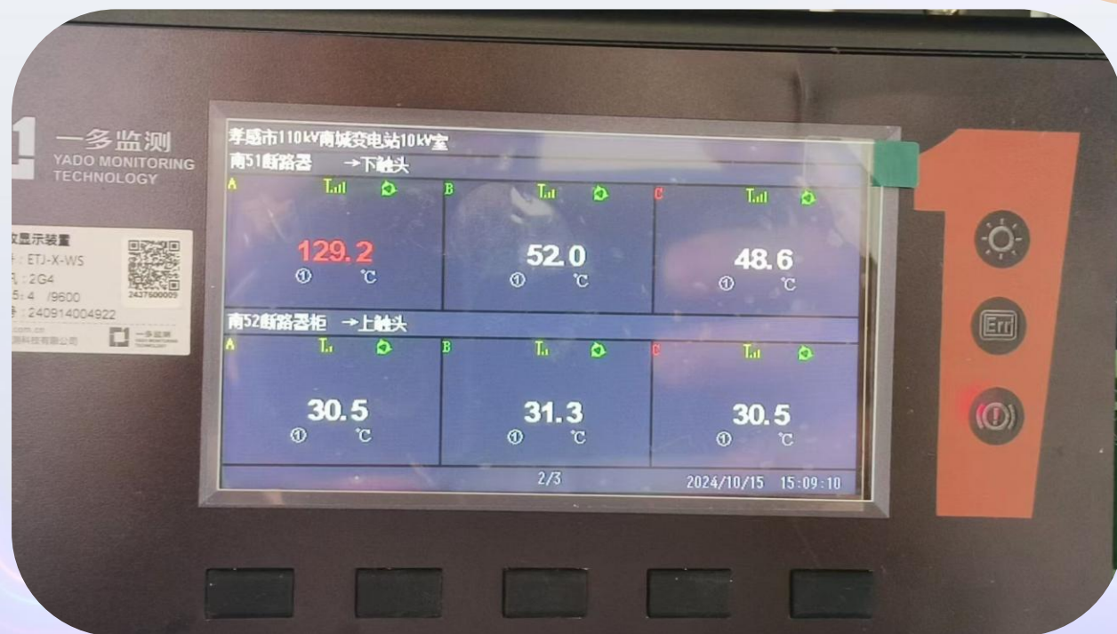
Overheating Emergency ALARM
