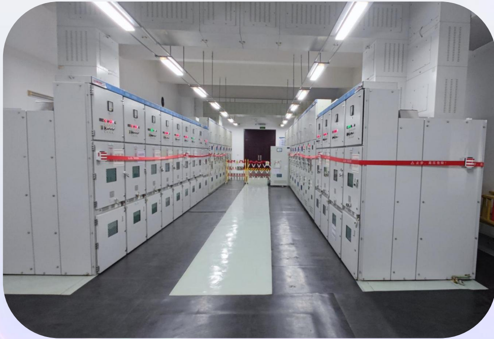
MV 10KV Switchgear Electrical Room of South City Substation in Xiaogan, Hubei, China
